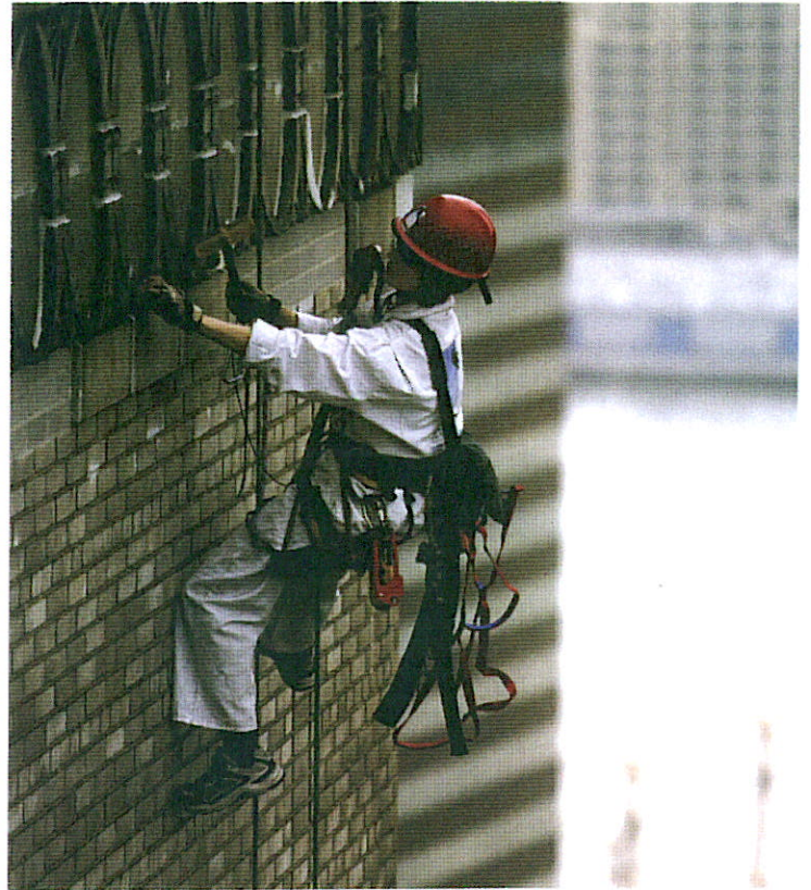
A surveyor, suspended by a two-rope system similar to that used by climbers, evaluates and documents facade conditions of a historic building.
